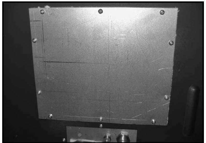
Figure 2: Access cover to valve control center.
