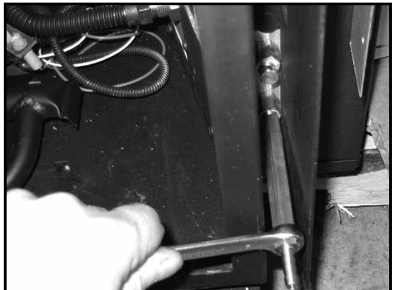
Figure 21: Attaching test extension.
