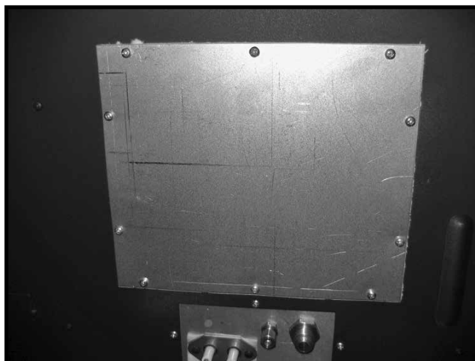
Figure 5: Access cover to valve control center.
