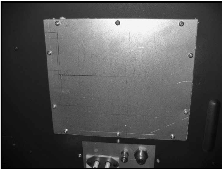
Figure 3: Access cover to valve control center.
