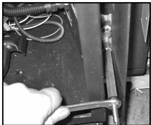
Figure 37: Adjusting manifold pressure.
