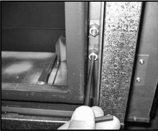
Figure 38: Removing manifold pressure plug.
