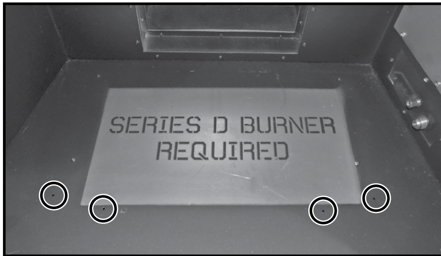
Figure 2: 4 holes in fireplace floor to be plugged.
