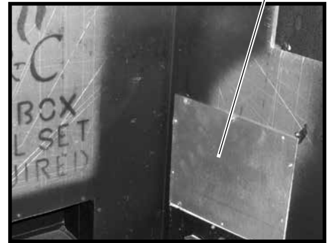
Figure 23: Access to firebox.
