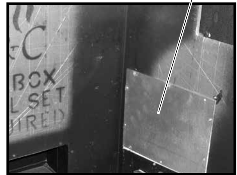
Figure 23: Access to firebox.
