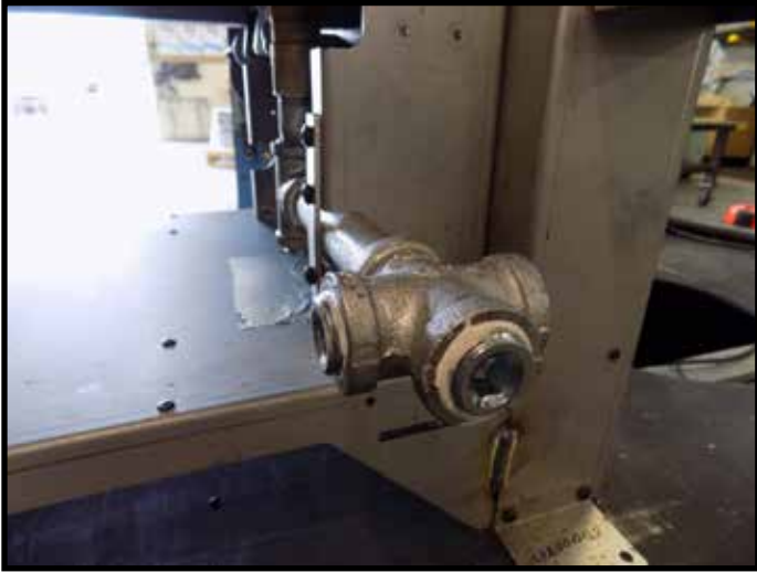
Figure 62: Gas connection point.
