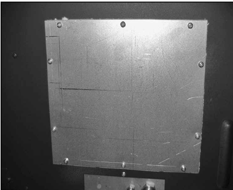
Figure 2: Access cover to valve control center.
