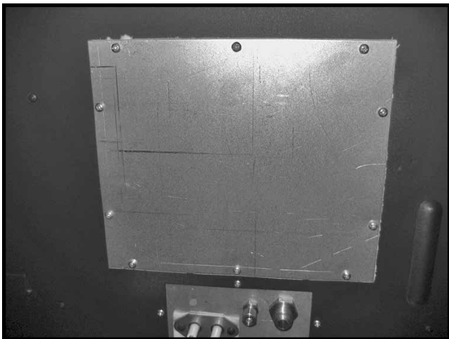
Figure 2: Access cover to valve control center.
