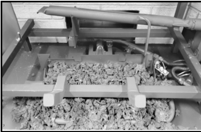
Figure 20: Ember material on lower burner.
