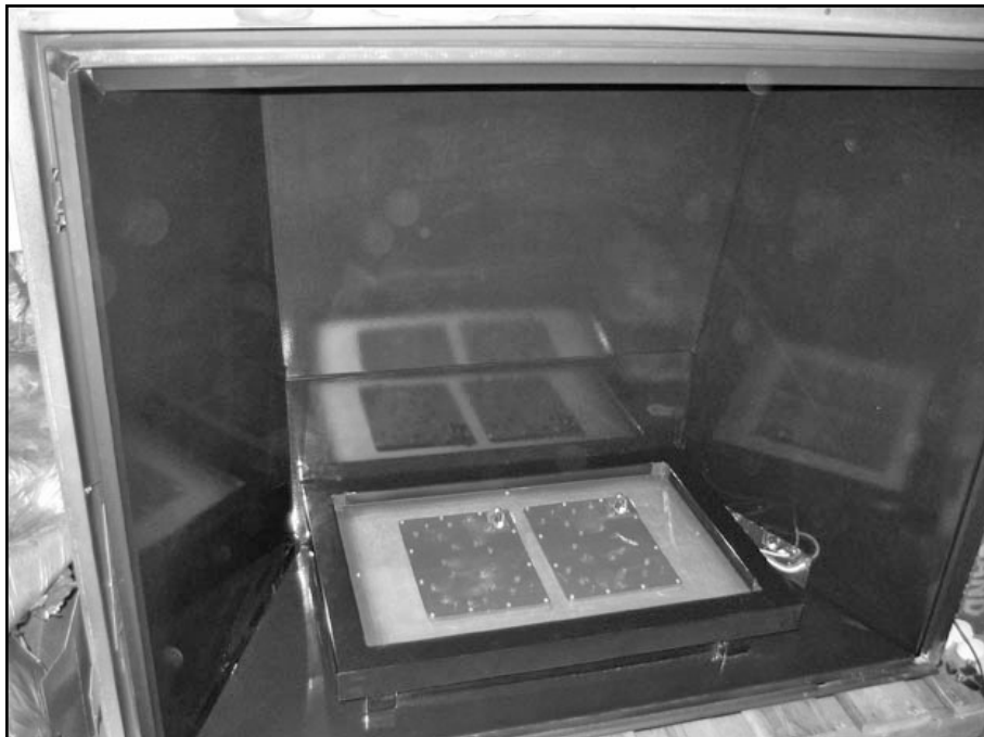
Figure 9: Burner assembly installed.
