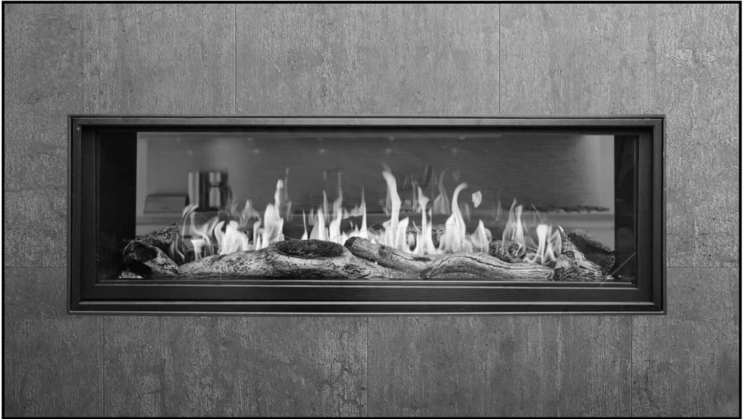
Figure 43: Example of desirable flame pattern.
