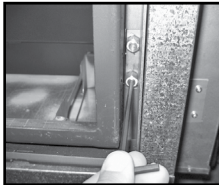
Figure 21: Gas pressure adjustment location.
