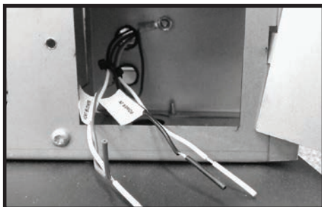
Figure 25: Junction box wiring.
