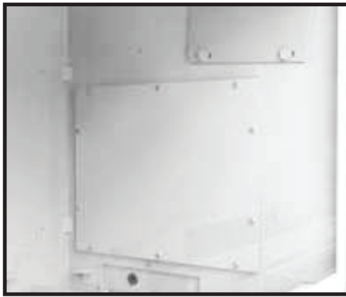
Figure 30: Gas valve cover.
