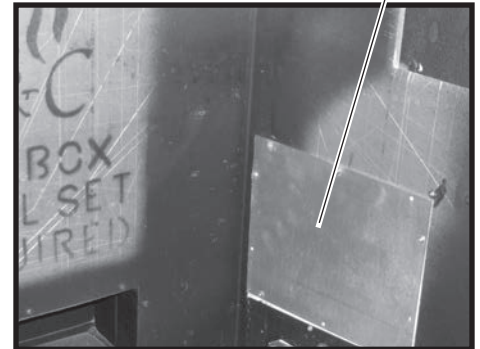
Figure 22: Access to firebox.
