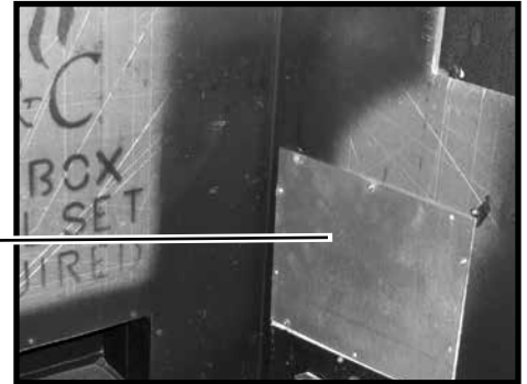
Figure 23: Access panel location.
