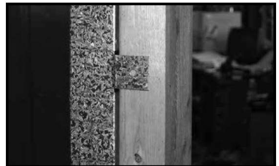
Figure 19: Framing tabs bent out.
