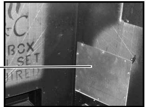
Figure 23: Access panel location.
