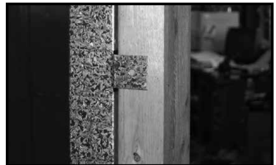
Figure 19: Framing tabs bent out.
