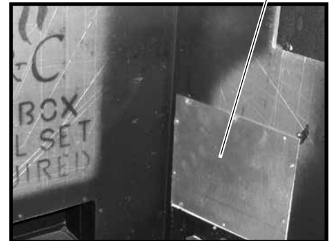
Figure 22: Access to firebox.
