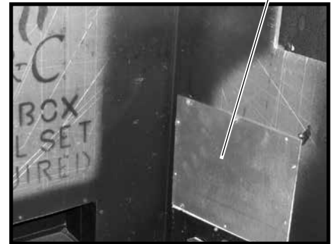
Figure 22: Access to firebox.
