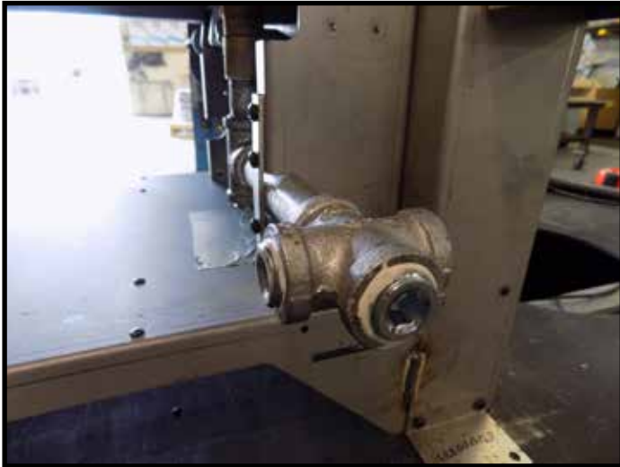
Figure 64: Gas connection point.
