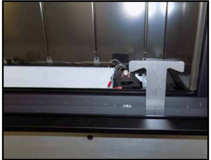
Figure 65: Gas valve shut off.
