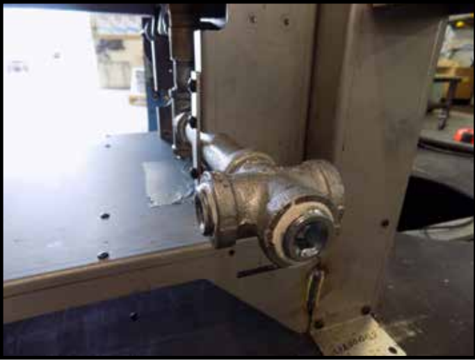
Figure 35: Gas connection point.
