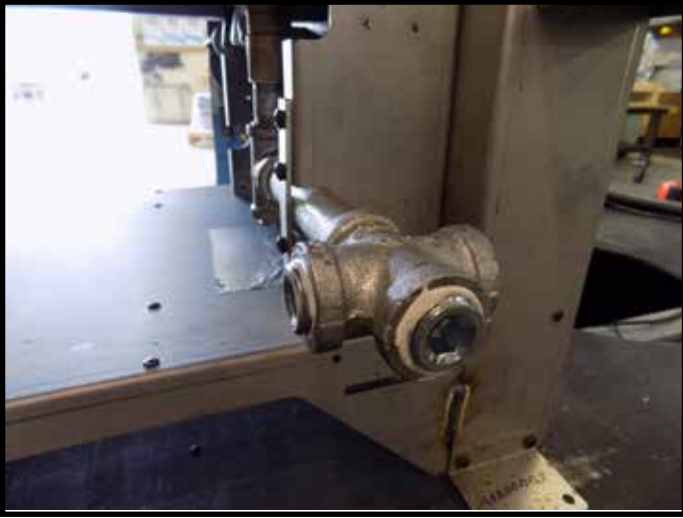
Figure 30: Gas connection point.
