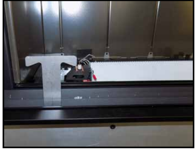
Figure 31: Gas valve shut off.
