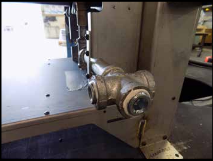
Figure 32: Gas connection point.
