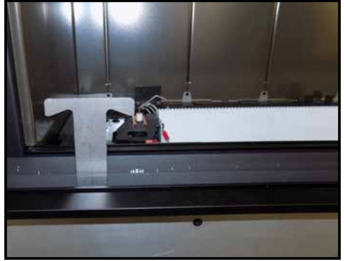
Figure 33: Gas valve shut off.
